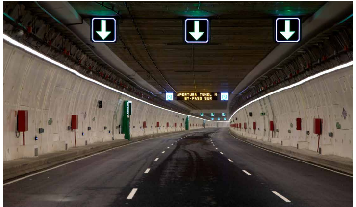
▲ M-30 Madrid (Spain): M-30 Southern Bypass, North Tunnel. Length: 4.156 km. Tunnel with two levels: one for traffic, the other for maintenance.
